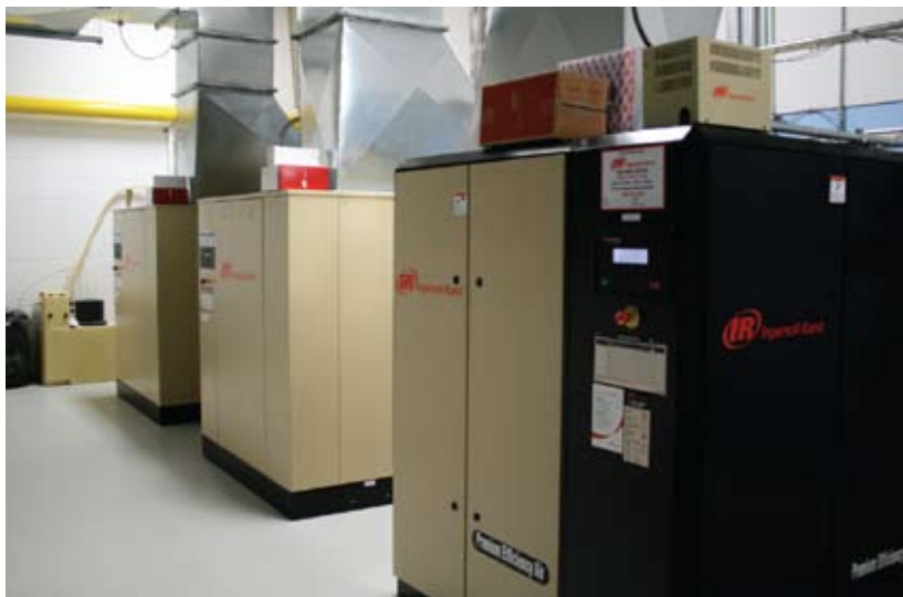
A view of three air compressors in the plant.
