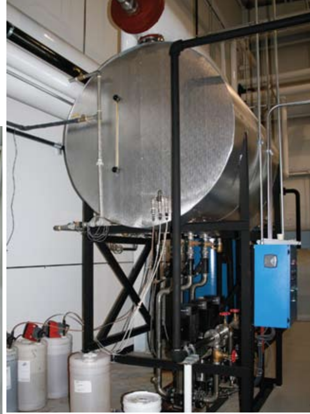
A view of the boiler makeup tank.
