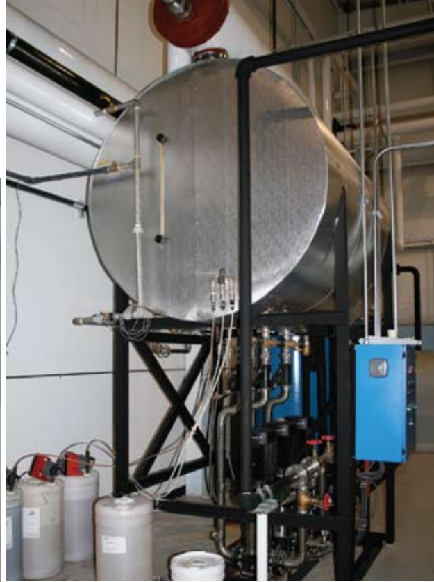
A view of the boiler makeup tank.
